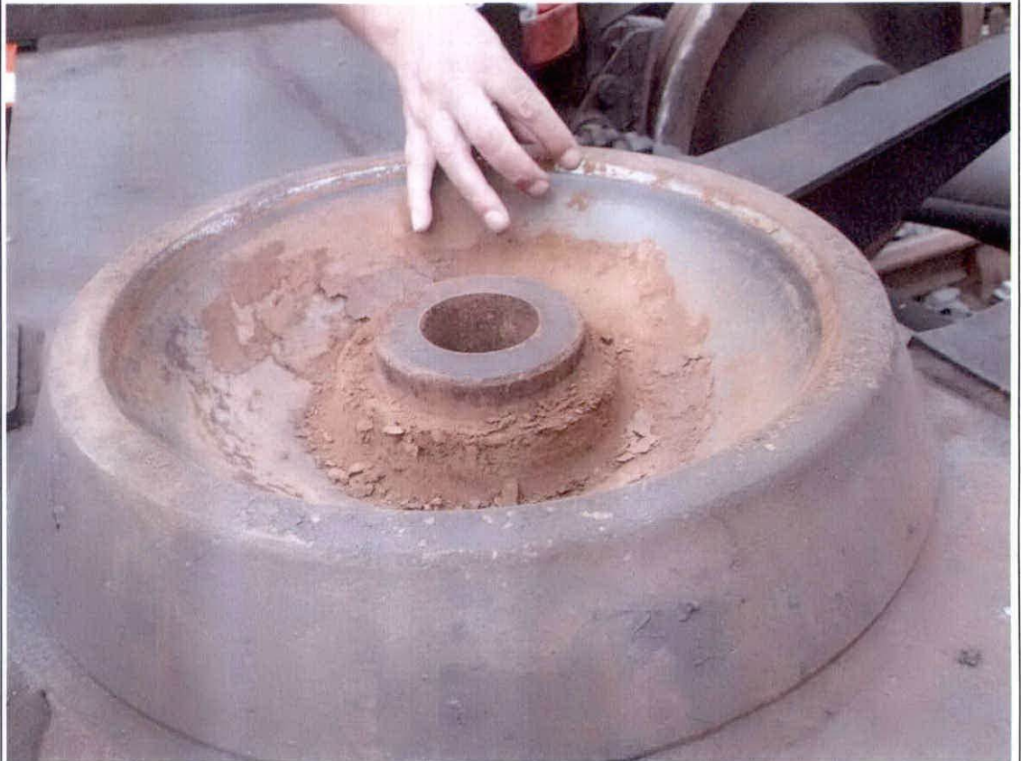
Figure 2: Centre pivot liner worn below level of steel rim, leading to contact between steel surfaces
