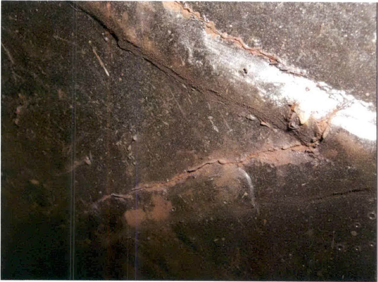
Picture 3 : Failed repair by welding
