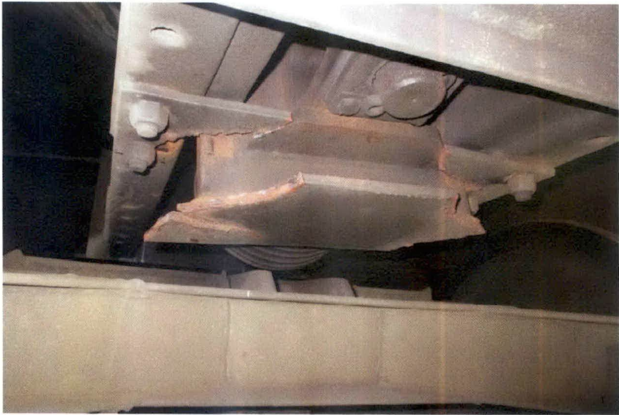
Picture 2 : Cracks in the baseplate - failure of the support bearing
