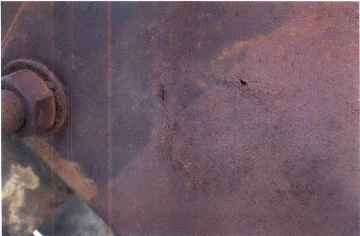
Picture 1 : Obvious tear in the baseplate
